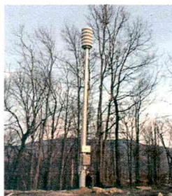
WARNING SIREN AT NORTH CLUBHOUSE
