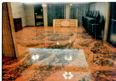
Water and debris from flood at North Clubhouse 2/20/15
